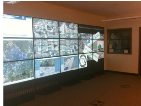
The video wall at the City of Gainesville Public Works – Traffic Management Center
