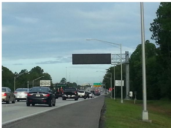
Coming soon to Butler Boulevard, A Dynamic Message sign westbound before Bowden.
