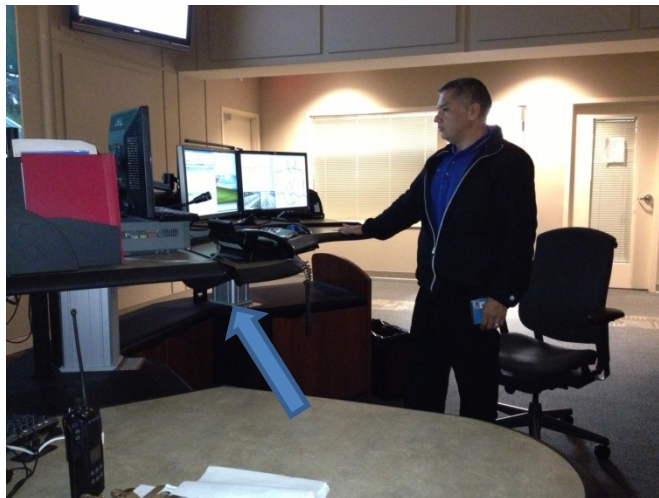
One of the TDOT Operators shows us their configurable workstations. The arrow shows the hydraulics, with cable chase, that allows the workstation to go from conventional desk height to a height to accommodate a standing Operator. Great for long shifts!
