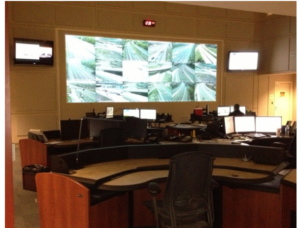
Inside the TDOT TMC Control Room (one of four TMCs Statewide)
