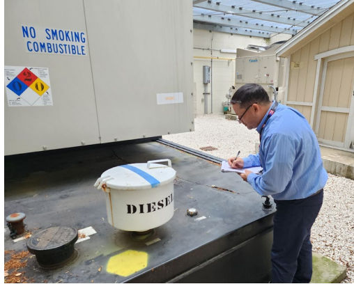
Generators and fuel ✓
